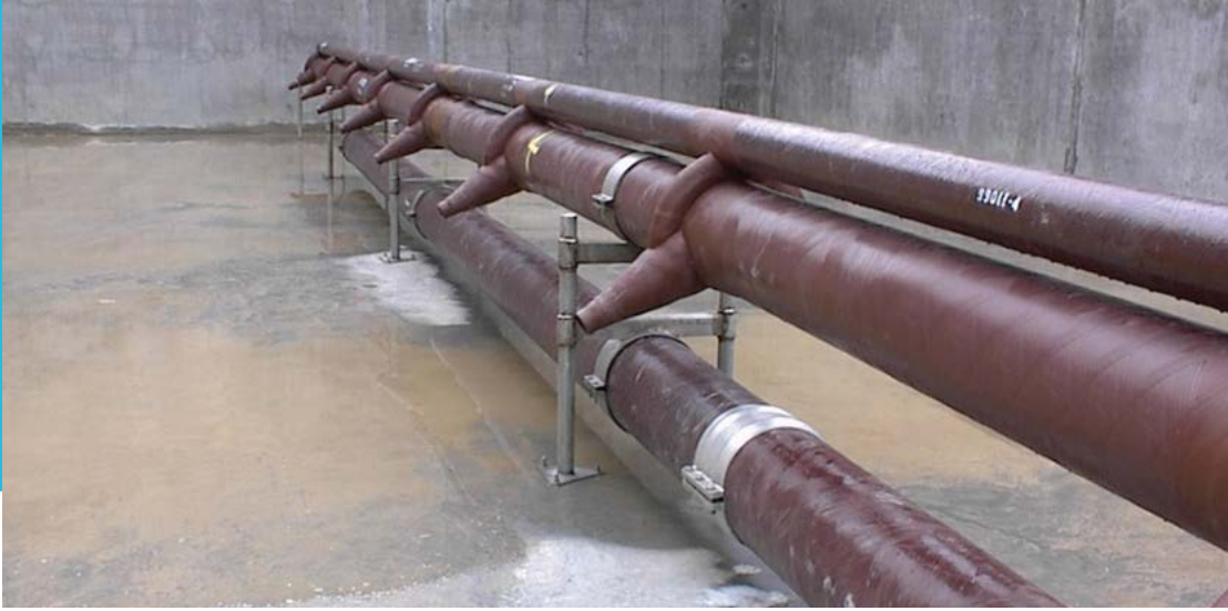
Influent distribution manifold
