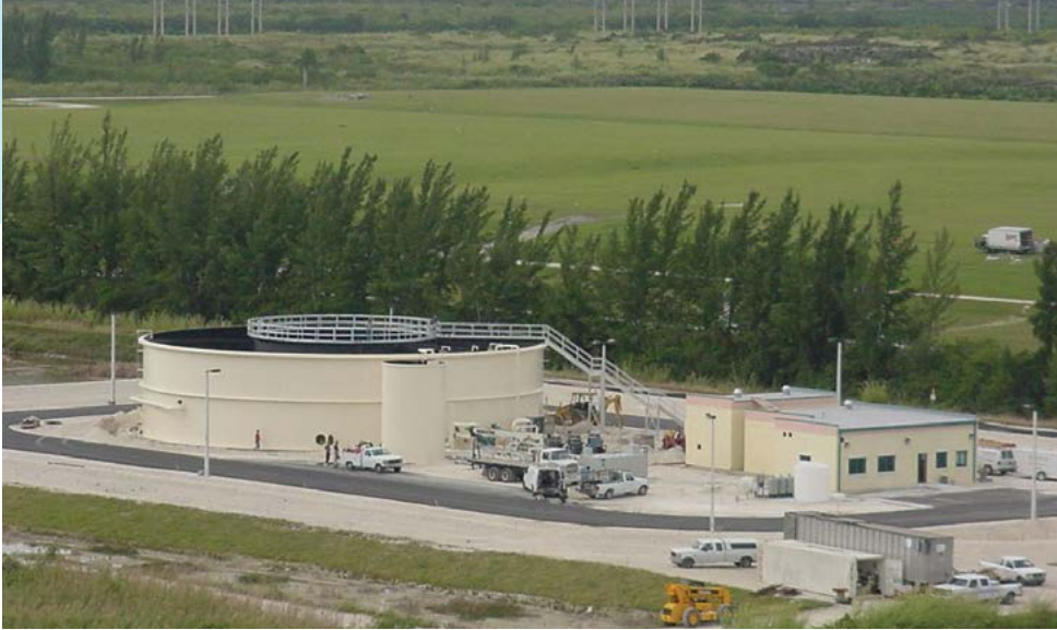
OMNIPAC® Field-Erected SBR system installed at municipal wastewater treatment plant
