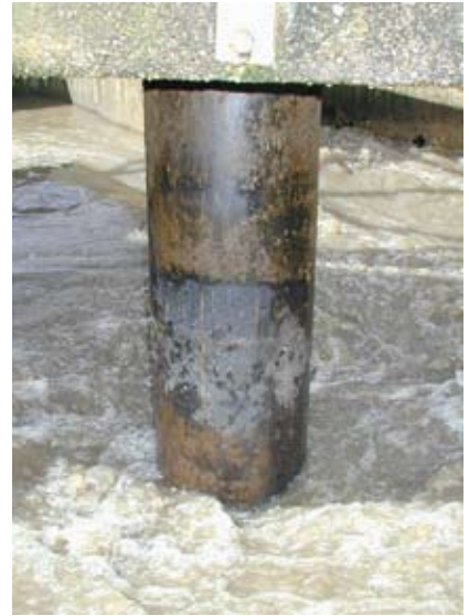
The effects of the continuous aeration can be clearly seen on the tank surface.
