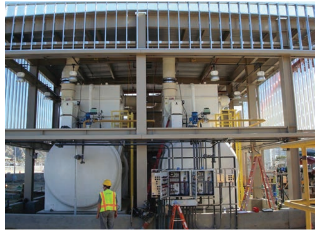
RJ-2000® Bulk Scrubber, Joseph Jensen WTP, Sylmar, CA
