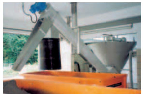
COANDA Grit Classifier discharging into a dumpster
