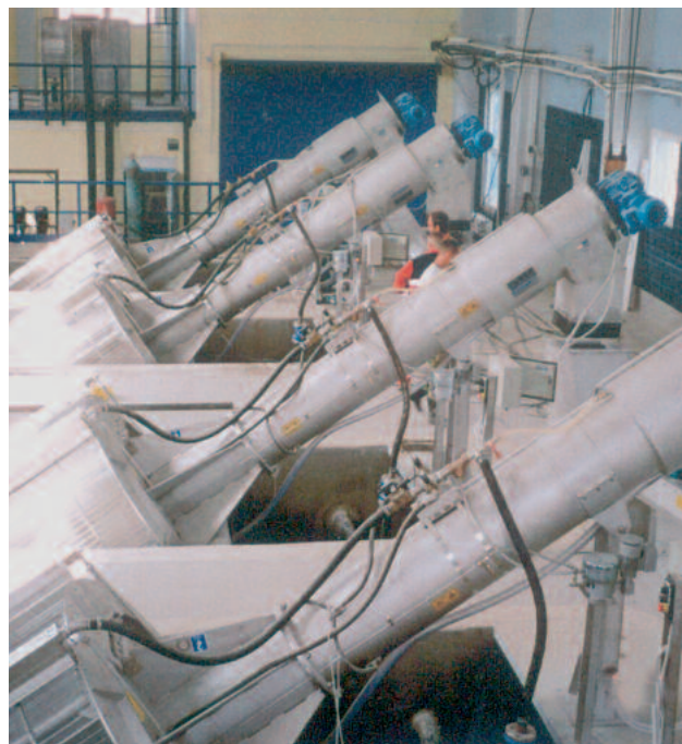
Four ROTAMAT® Rotary Drum Fine Screens provided with integrated screenings washing (IRGA)
