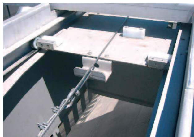
Semi-automatic grease removal by means of a paddle system
