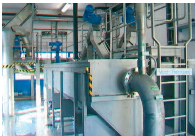
Above-ground redundant installation of a HUBER Grit Trap Ro6
