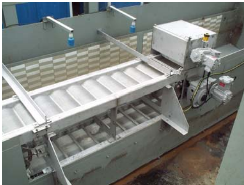
Wilmslow, UK 14, mgd (600 l/s)
