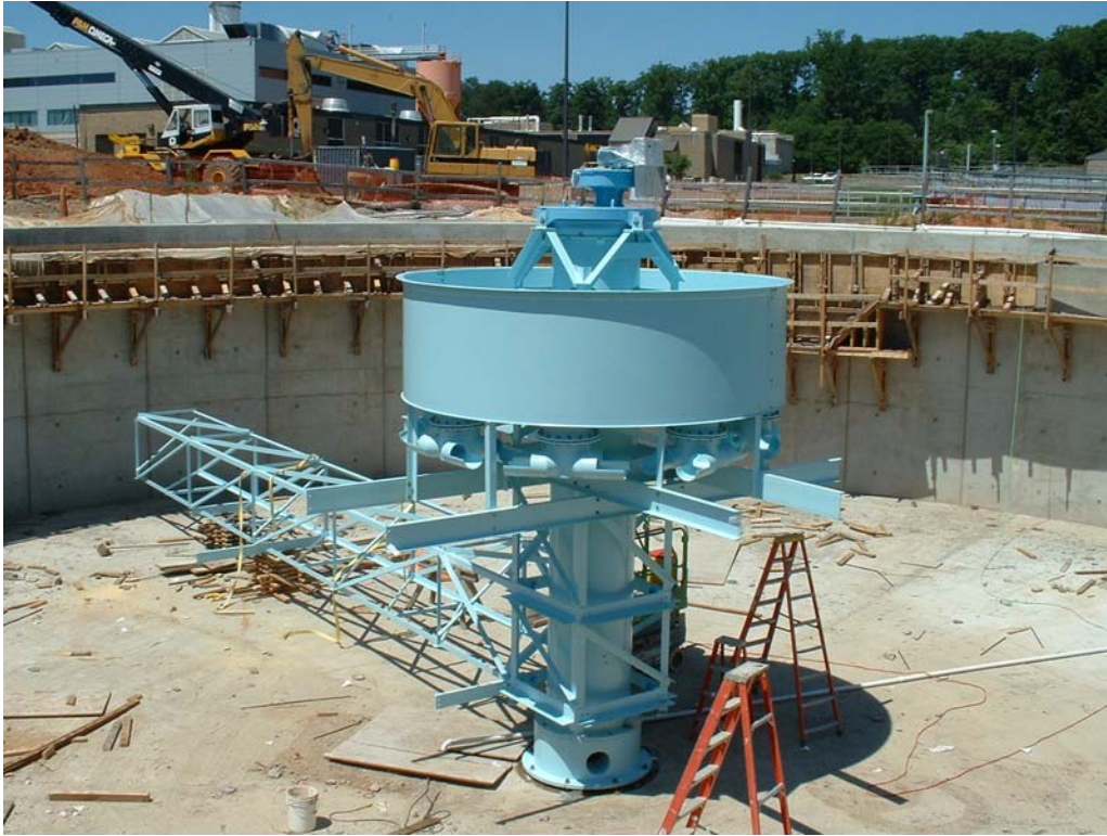
Figure 1: Energy Dissipating Inlet (LA-EDI)
