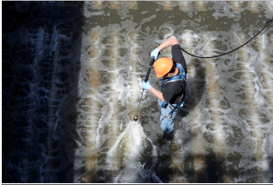
Figure 5. A worker pressure washing the 12-year old diffusers in the north tank in 2013. It took 3-4 hours to pressure wash the entire tank.
