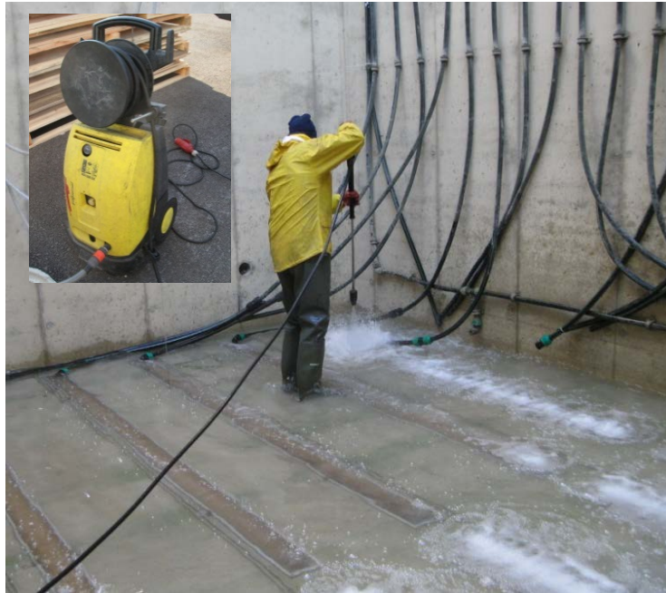
Figure 4. Pressure washing the eleven-year old diffusers at the factory test tank in 2012. The positive effects of pressure washing can be seen on the air distribution pattern.
