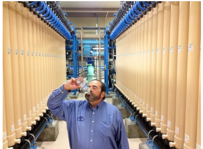
Hendersonville Utility District General Manager Tom Atchley drinks water bottled at their treatment plant.
